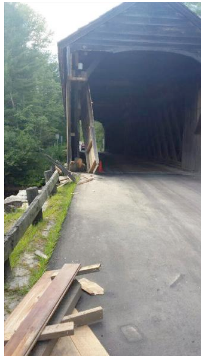
The Corbin Covered Bridge in Newport will be closed for this week for repairs. The bridge was damaged by a hit and run driver in August (File photo).
