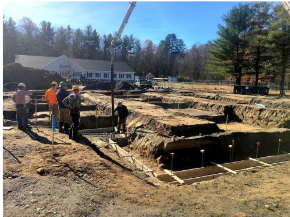
Workers were busy pouring cement this Monday morning for the footings of the new National Field Representatives building project on Maple Ave. in Claremont. They were expected to install the cement for the new crosswalk lights today as well (Courtesy photo).
