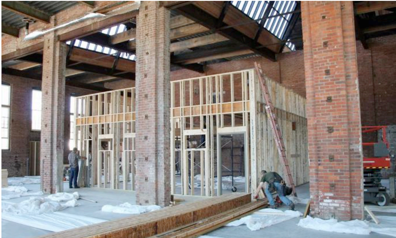
The cement floor has been poured at the MakerSpace (Sawtooth) building, and construction of the rooms has begun (Bill Binder photo).
