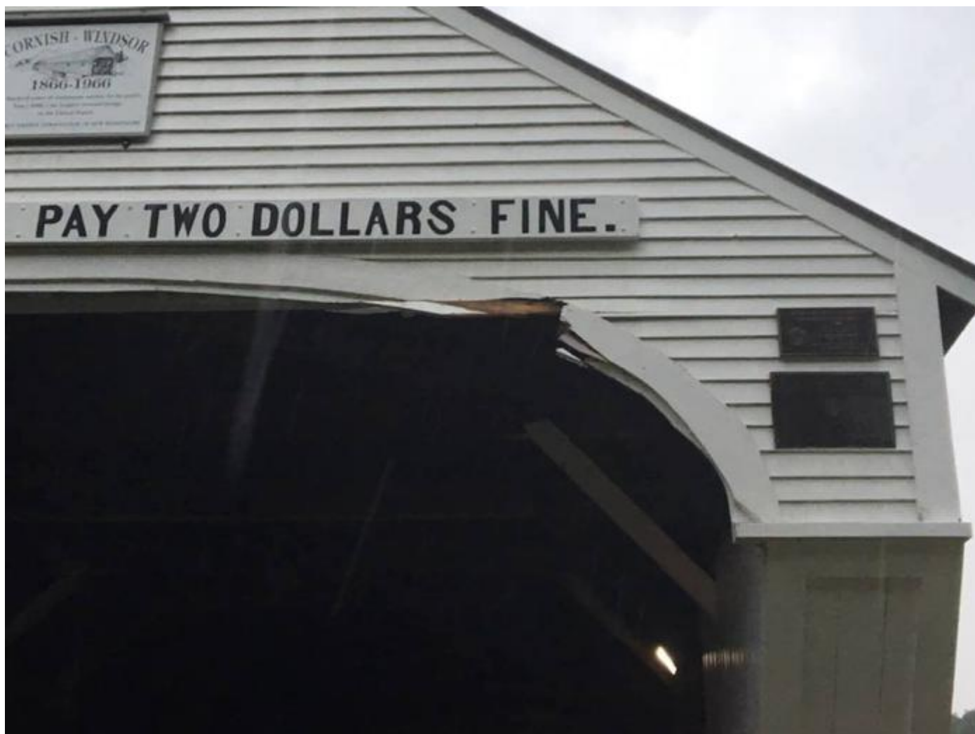
This is the second time in less than a month the historic Cornish-Windsor Bridge has been struck by a large truck attempting to cross the bridge (NH Dept. of Transportation photo).
