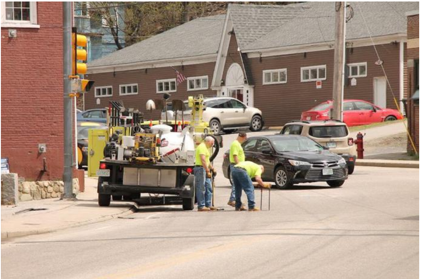
DPW workers in Claremont were out marking and locating water shutoffs and marking the road last week for the start of the Main St. project which begins today, Monday. Residents are reminded to seek alternate routes (Bill Binder photo).
