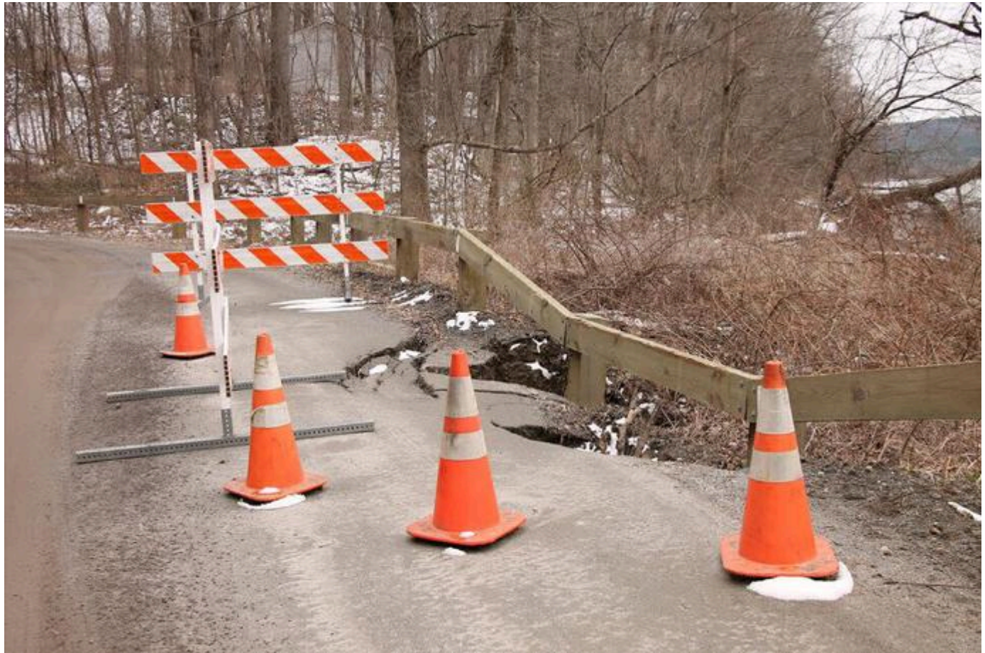
Heavy rains last week washed out a portion of a culvert under Ferry Landing Road in Claremont just around the turn at the bottom of the hill (Bill Binder photo).
