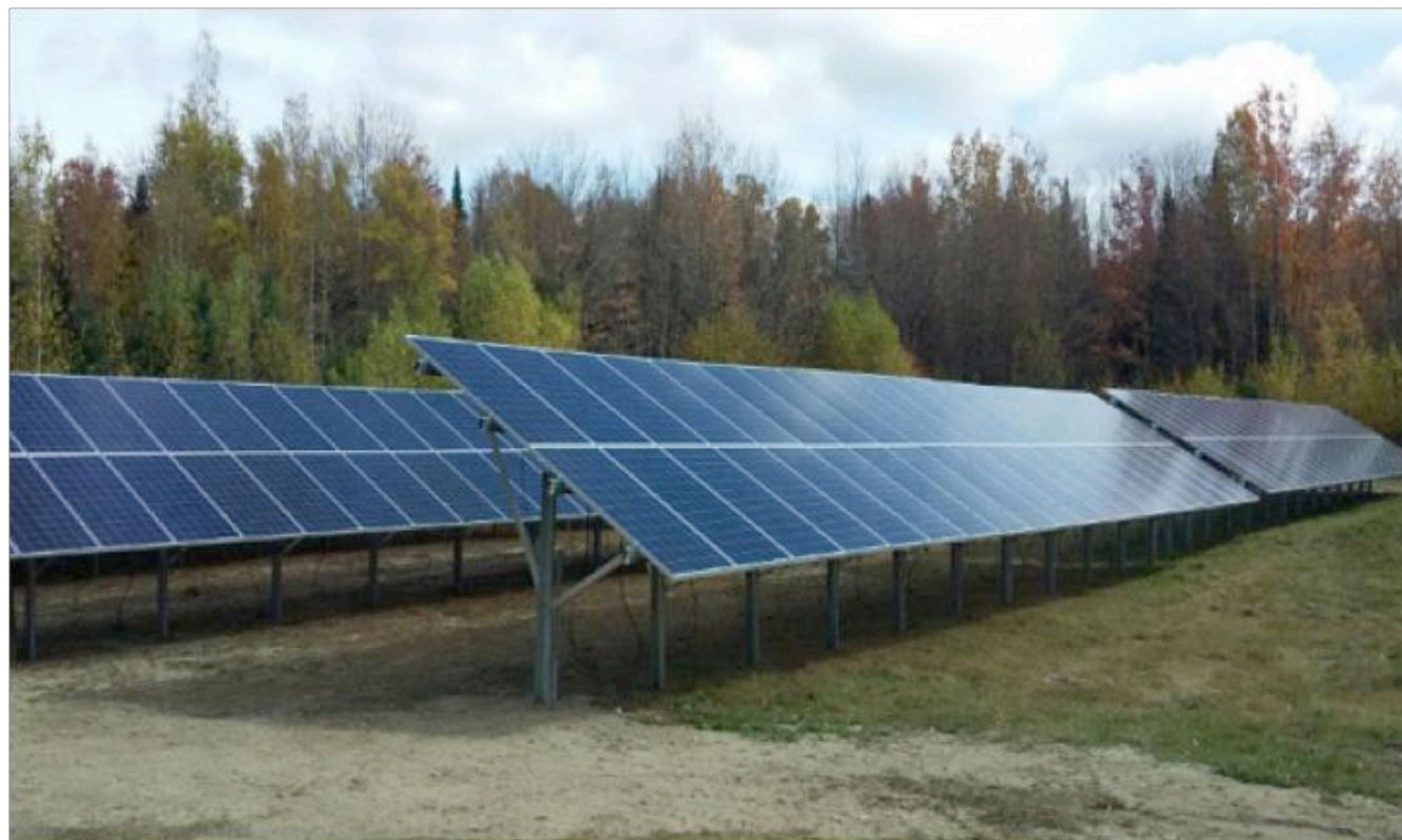
Sample ground mount solar array
