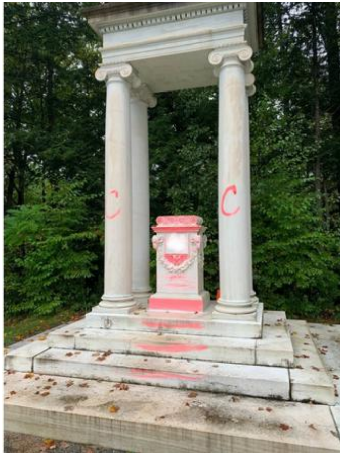
Image of the front elevation of the Temple at Saint-Gaudens National Historical Park, October 1, showing evidence of vandalism. (NPS photo).
