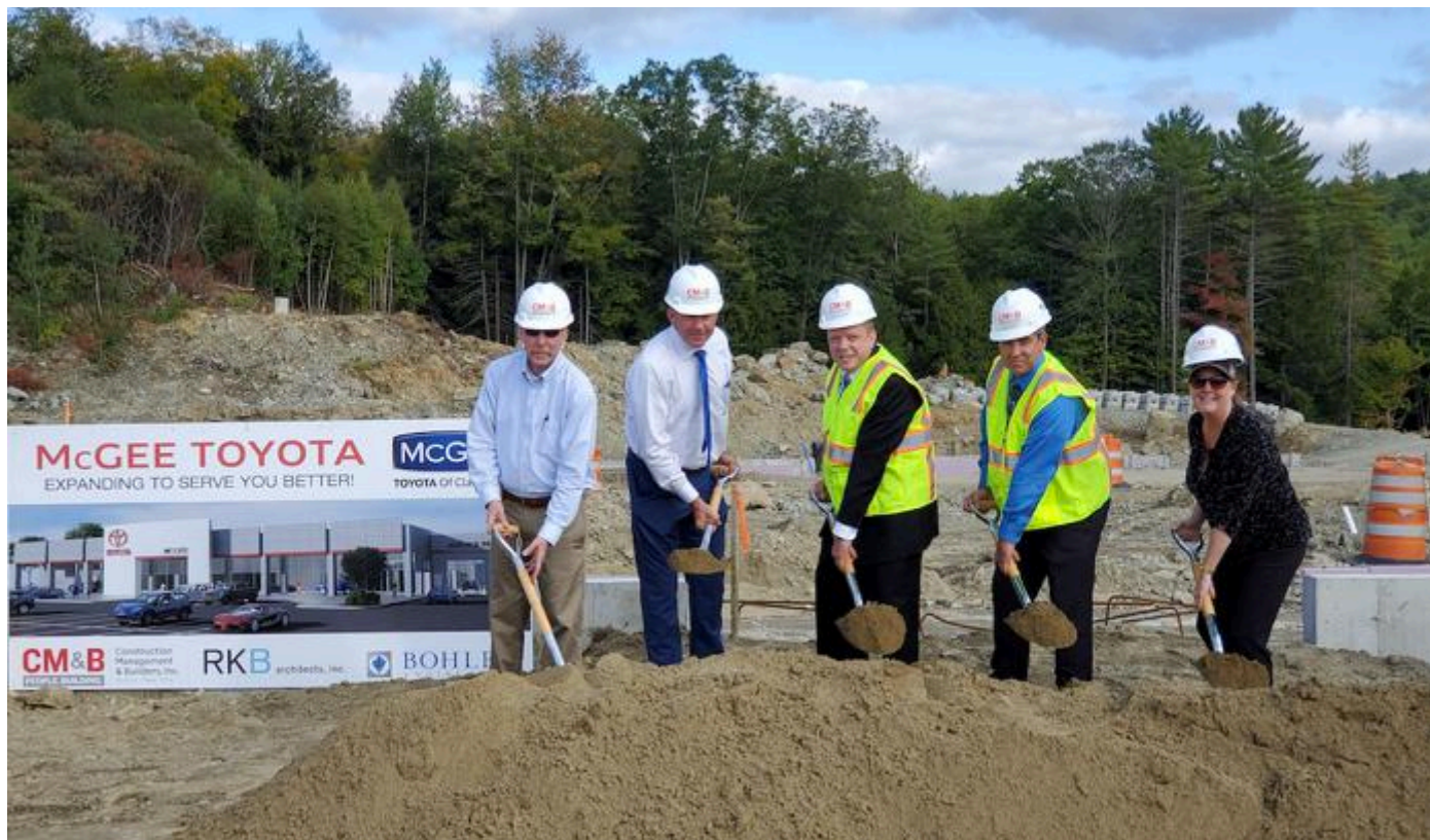
The McGee Toyota of Claremont management team shovel-start the project. From left: Parts manager Ken Everitt, general sales manager Chris Walker, general manager Phillip Gregoire, service manager Evan Roberts, and comptroller Anne Seward (Eric Zengota photo).
