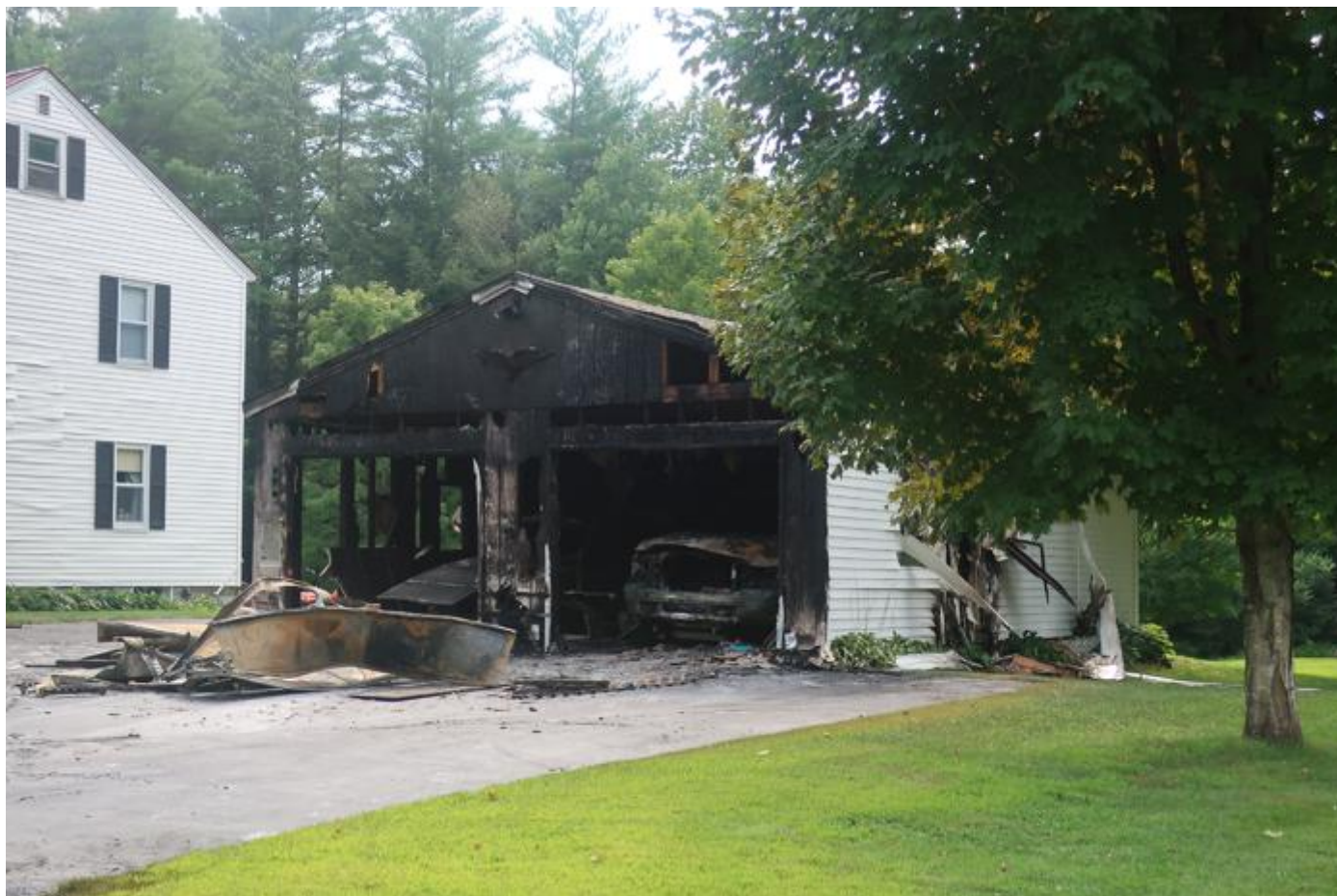
A two-car garage and its contents in Claremont were destroyed Thursday afternoon. Heat from the fire caused moderate damage to some of the siding on the house (Phyllis A. Muzeroll photo).
