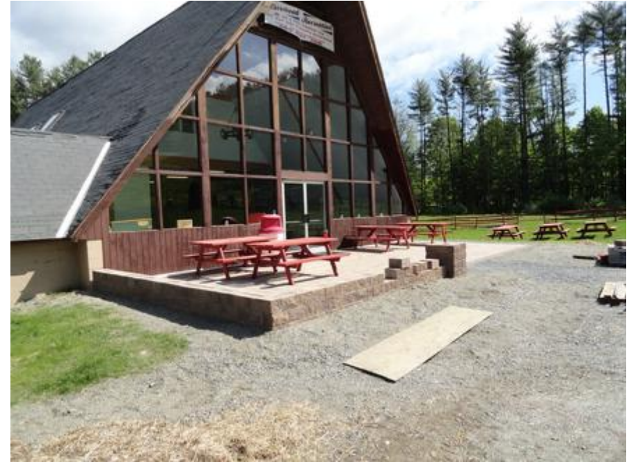
Work has been continuing on the patio short wall being built in front of the Arrowhead Lodge building (Courtesy photo).
