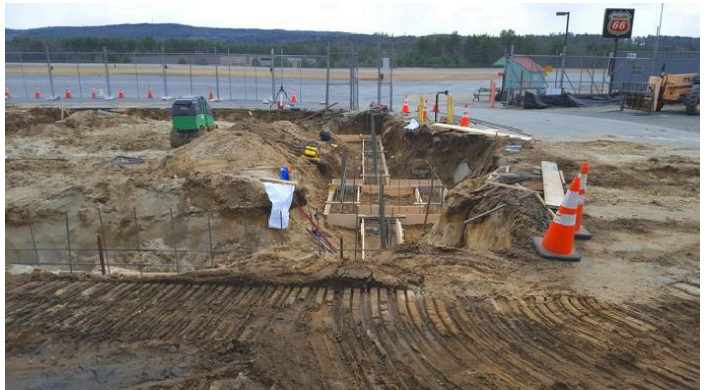
Pine Hill Construction began pouring the concrete footing for the new terminal last week (Courtesy photo).
