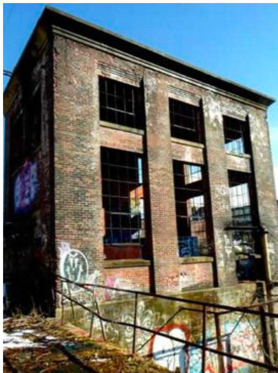
The condition of the powerhouse was described as ranging from fair to good.
