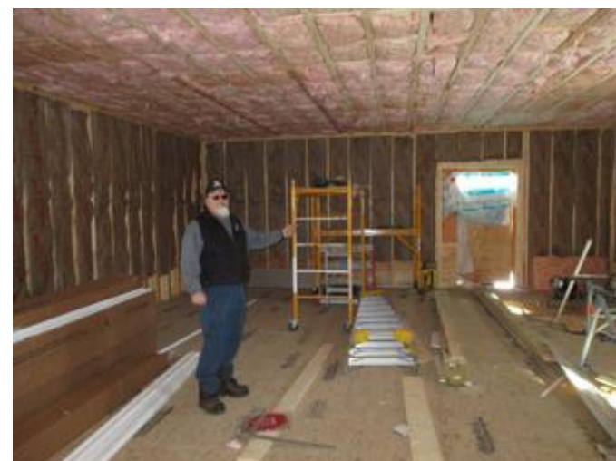
Top: Work is continuing on a new Lempster Post Office. Bottom: Daryl 'Bubba' Simino points out the need for plumbing and electrical wiring by the sub-contractors (Bill Murgatroy photos).
